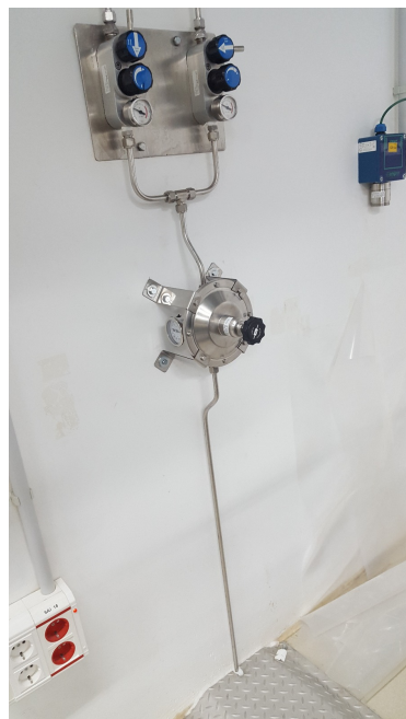
Figure 22. ATEKO-Air main line in Hall C.
